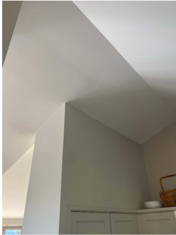
Minor cracks within the internal entry foyer and adjacent to the kitchen.
