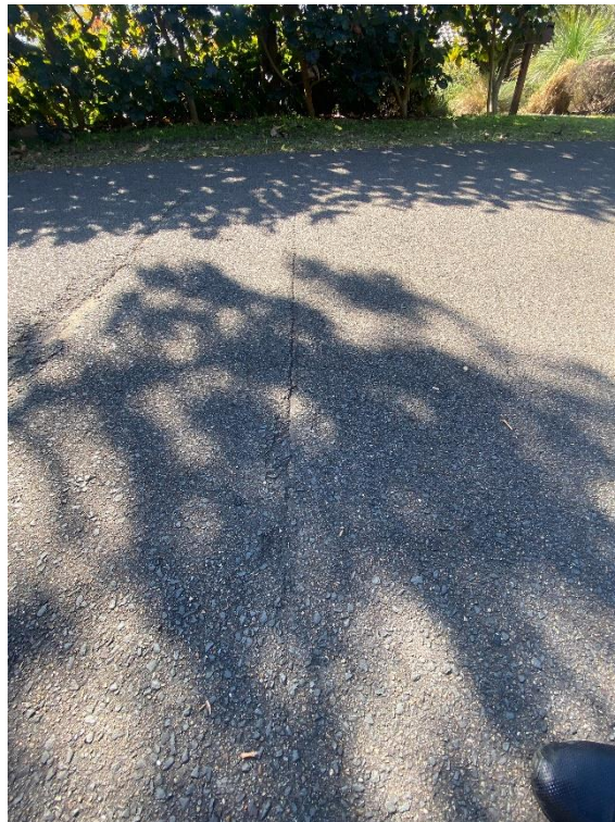
Cracks within the concrete / bitumen road in front of the proposed development site.
