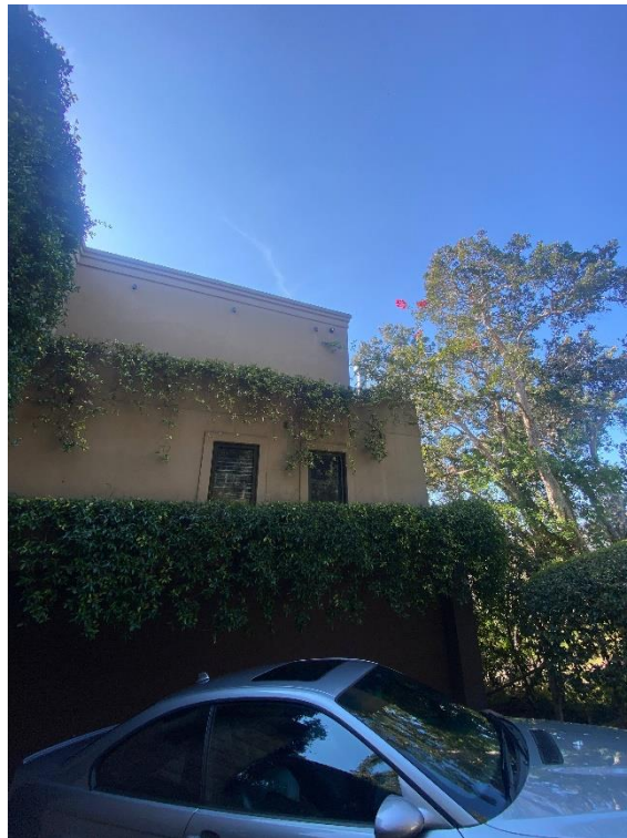
External front right corner masonry / rendered wall has a long splayed crack adjacent to the CCTV camera.
