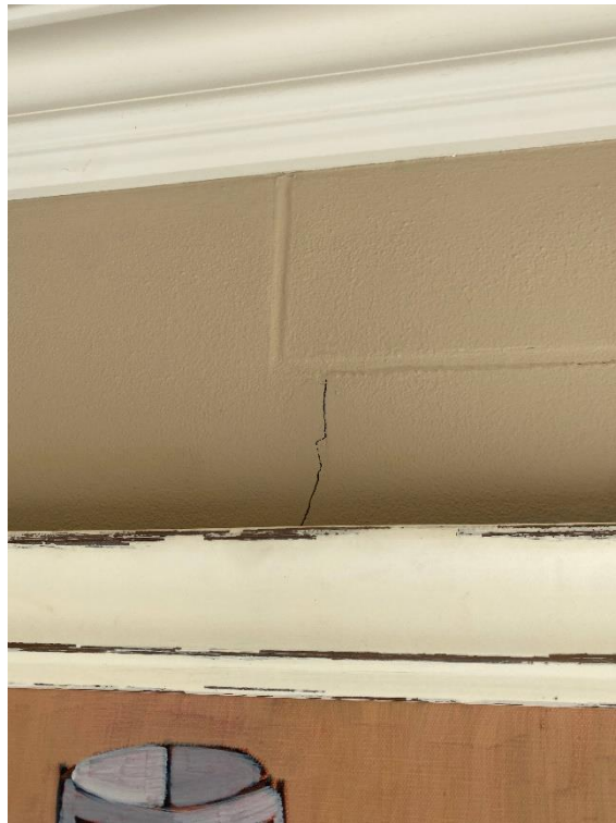
Minor cracks within the internal rendered walls beneath the cornices spanning behind the artwork.
