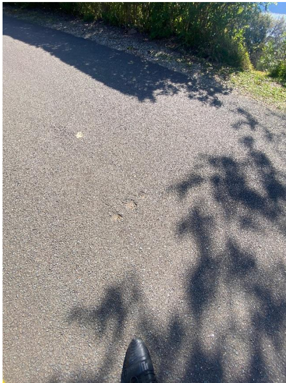
Cracks within the concrete / bitumen road in front of the proposed development site.
