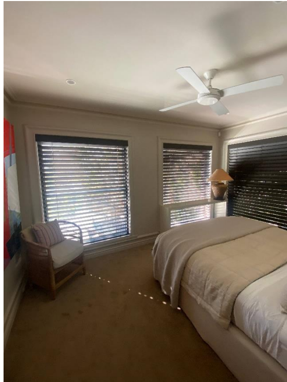
Internal bedroom has minor cracks within the rendered walls, I'm referring to the walls facing the rear of the property due north.
