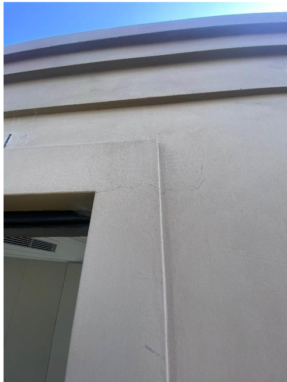
External walls of the home have minor hairline cracks within the right side external veranda.
