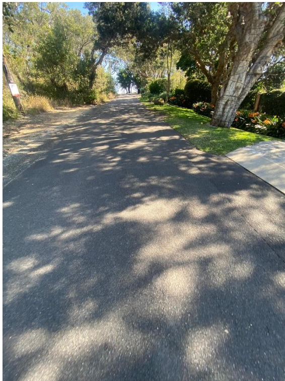
Minor cracking within the road.
