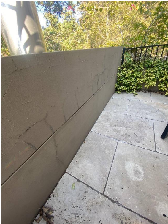
Outside veranda masonry walls have minor crazed cracking.
