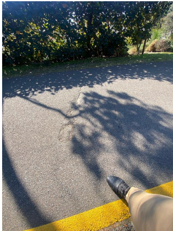
Cracks within the concrete / bitumen road in front of the proposed development site.
