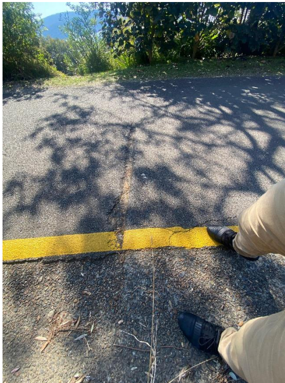
Cracks within the concrete / bitumen road in front of the proposed development site.
