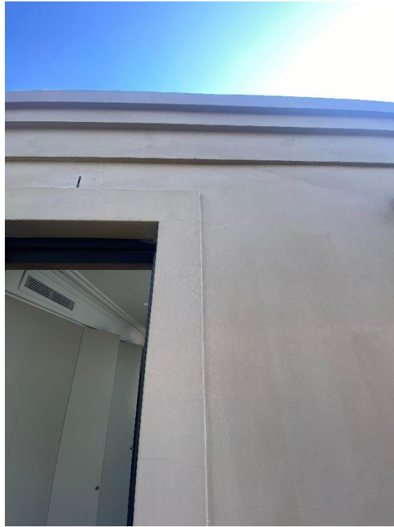
External walls of the home have minor hairline cracks within the right side external veranda.
