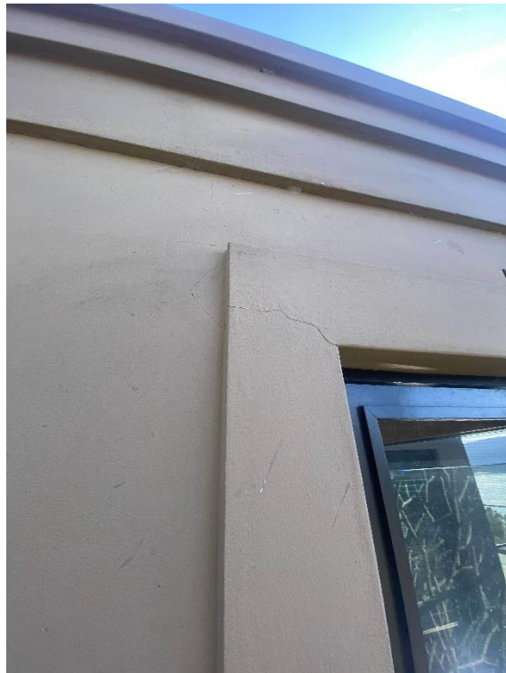
External walls of the home have minor hairline cracks within the right side external veranda.
