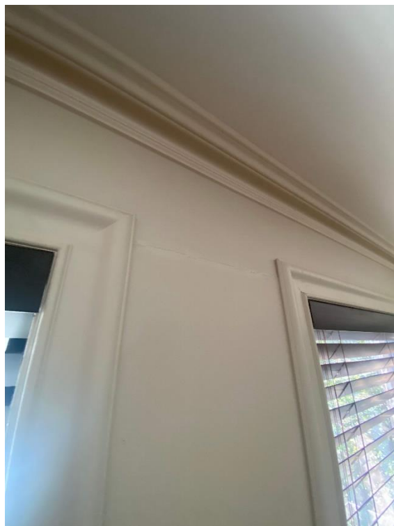
Minor horizontal cracks seen within the rendered walls between the windows.
