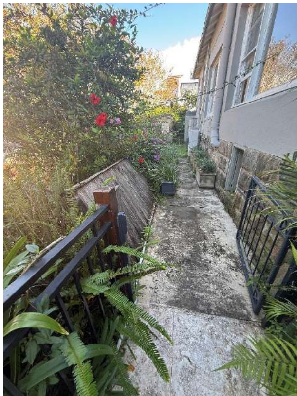
Boundary fence collapsed
