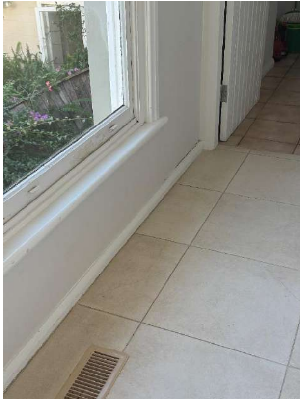
Vertical crack beneath the window within the wall below the double hung window
