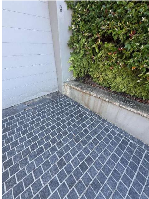
Minor cracks seen within the masonry boundary wall abutting the garage wall
