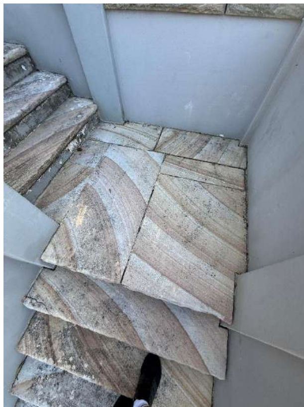
Minor cracks seen within the sandstone flagging floor tiles
