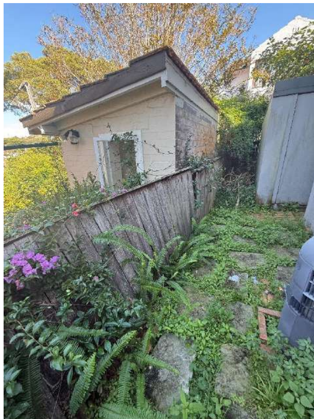
Collapsed boundary fence
