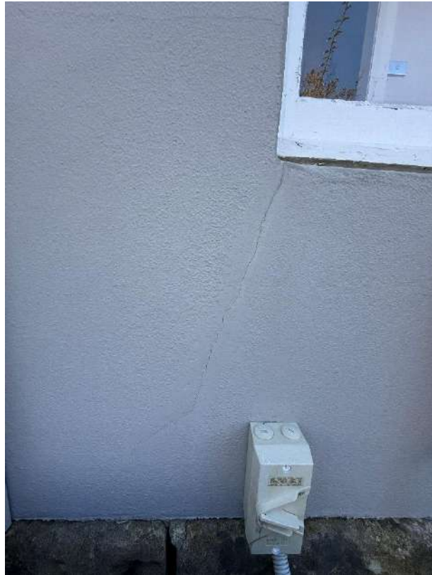
Horizontal and vertical cracks in the masonry wall to the bottom-left of the window
