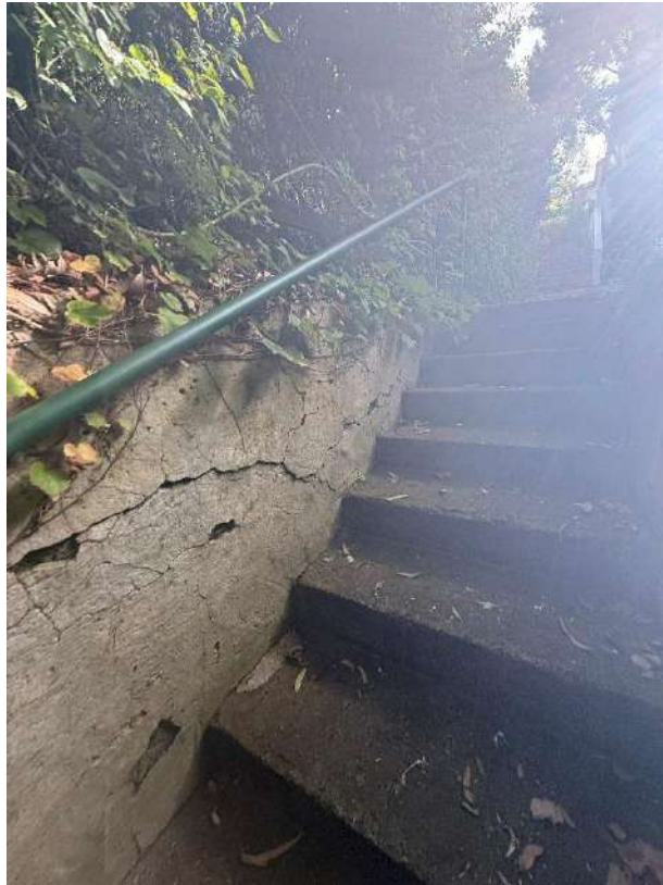
Left and right masonry walls on either side of entry stairs are structurally cracked horizontally and vertically within the masonry walls
