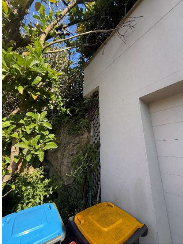
Top-left corner, minor hairline cracks within the masonry wall abutting the sandstone boulder
