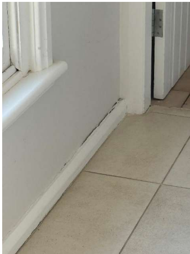
Crack within the timber skirting board within the junction in the hallway
